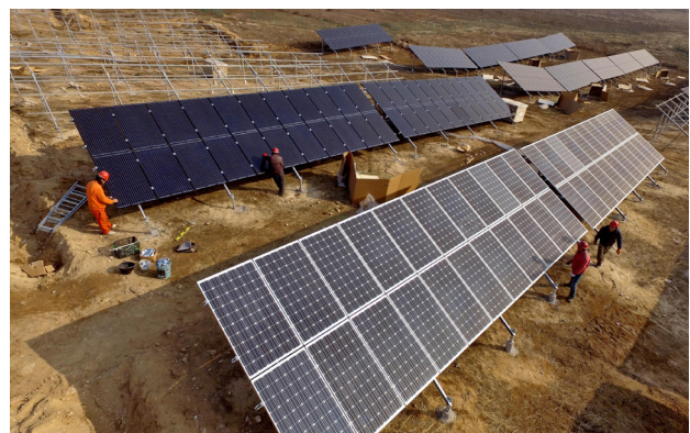
Installing solar panels in rural areas of Hebei province, as part of a 2015 nationwide poverty alleviation project. African countries struggling to electrify their power grids could learn from China’s experience in achieving universal energy access. (Image: Yang Shiyao / Alamy)
